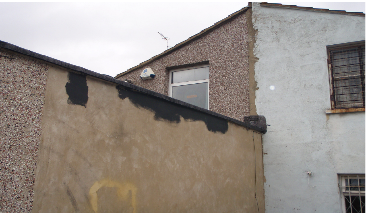
The flat roof area is the roof of the rear room area of the premises. The first floor is a commercial office property.
